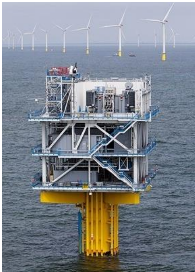
London Array Substation on monopile Photo Credit: Siemens Press
